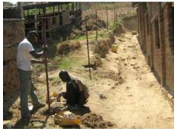
Above is the Fence being built at Fruits of Hope Academy with funds raised by Inaburra Pre-School and Inaburra Global Education team.
